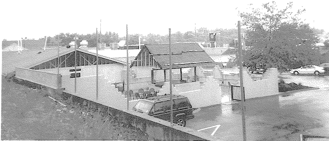
VIEW FROM MY DRIVEWAY LOOKING AT THE PARTIALLY COMPLETED COVERED BAR AND PATIO AREA
