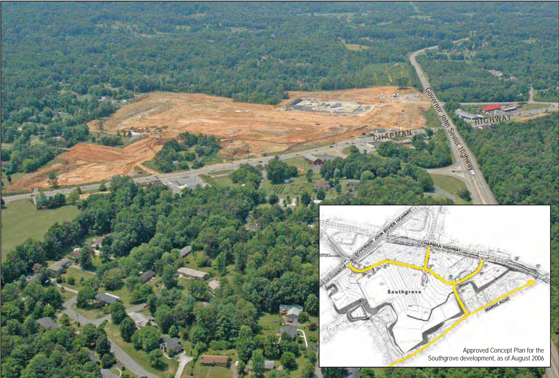
This aerial view of the Governor John Sevier Highway interchange shows the 40-acre construction site of Southgrove, a new commercial development. The James White Parkway extension is expected to intersect with Chapman Highway somewhere in the general area, and it is important that a location be identified to preserve the right-of-way from continued development.
