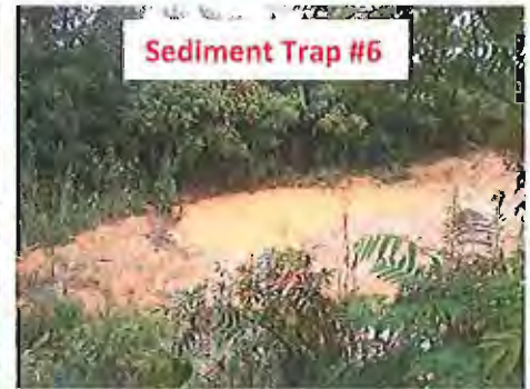
This trap is virtually no available storage; therefore it is not functioning property. Additional volume should be created.
