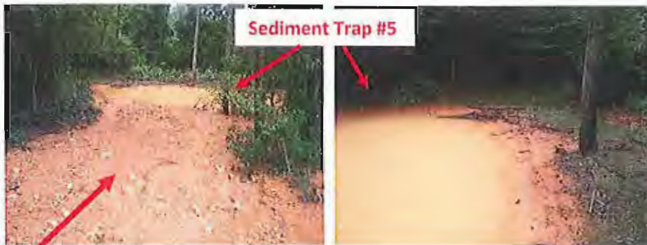
This sediment has washed into the sinkhole and must be removed.
