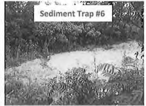
This trap is virtually no available storage; therefore it is not functioning property. Additional volume should be created.
