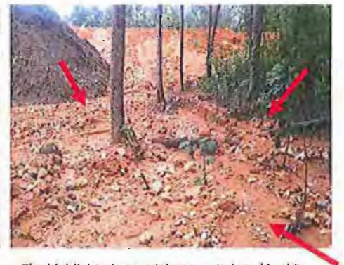
The highlighted material was not placed in this area, but has washed out from the fill area above.
