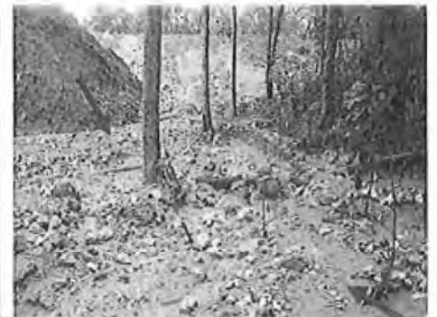
The highlighted material was not placed in this area, but has washed out from the fill area above.
