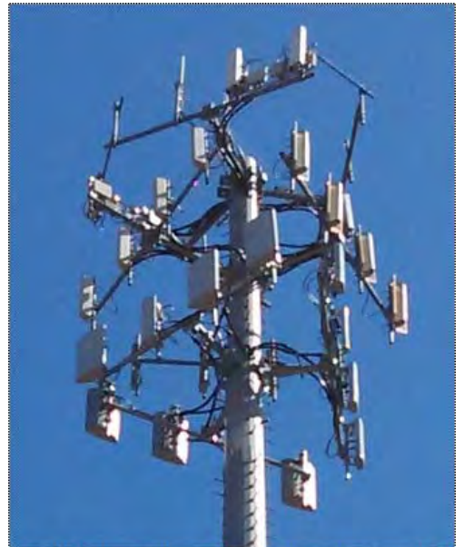
Cell Phone Tower Antenna array in Kent NY.
