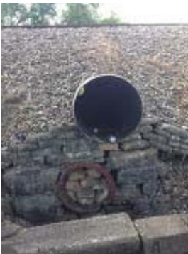
Drain pipes on to propose development.JPG 522K
