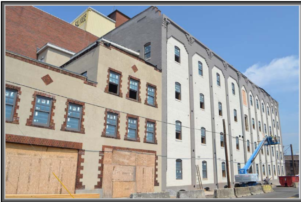
View of the White Lily Building from N. Central Street - façade restoration in progress.
