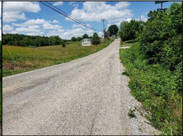
Steep road/shoulder drop-off and deteriorated pavement near 701 Brakebill Road Driveway (Looking North)
