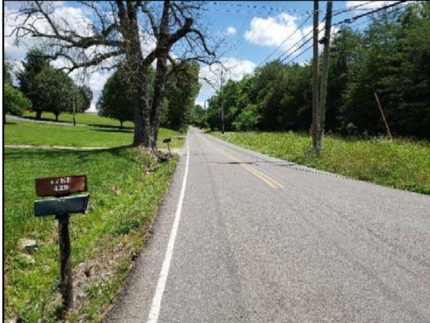
Large trees and utility poles adjacent to the roadway near 428 Brakebill Road with shoulder drop-off into the drainage ditch (Looking South)
