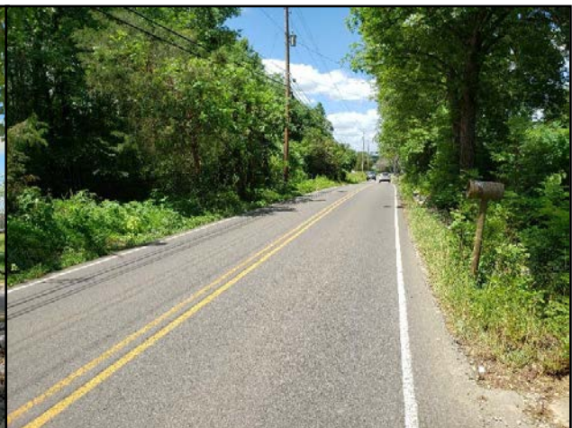
Large trees and utility poles adjacent to the roadway near 508 Brakebill Road with shoulder drop-off into the drainage ditch (Looking North)
