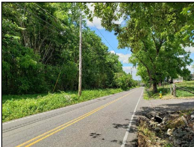
Large trees and utility poles adjacent to the roadway near 512 Brakebill Road with shoulder drop-off into the drainage ditch (Looking North)
