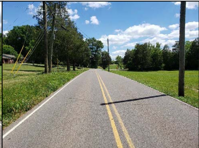
Utility poles adjacent to roadway near 322 Brakebill Road with shoulder drop-off (Looking South)
