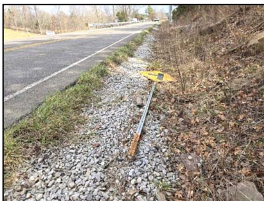
Knocked Down Side Road Sign on Strawberry Plains Pike
