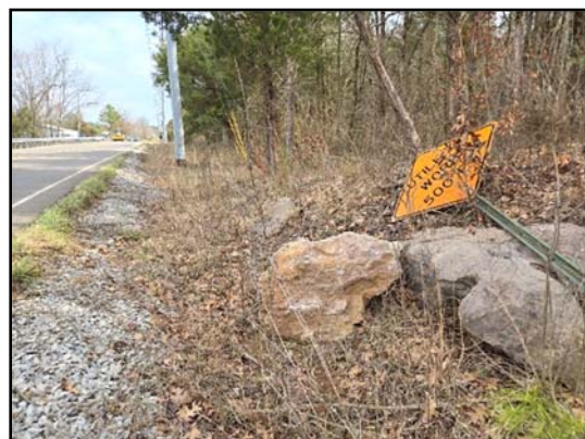
Knocked Down Construction Sign on Strawberry Plains Pike
