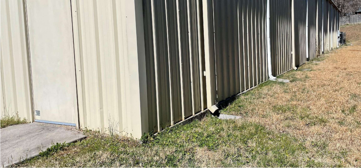
Figure 19 - 2725 Shipetown Rd Dollar General – None of the required 4' planting around 50% of building exterior (there is none on the front or other sides either)
