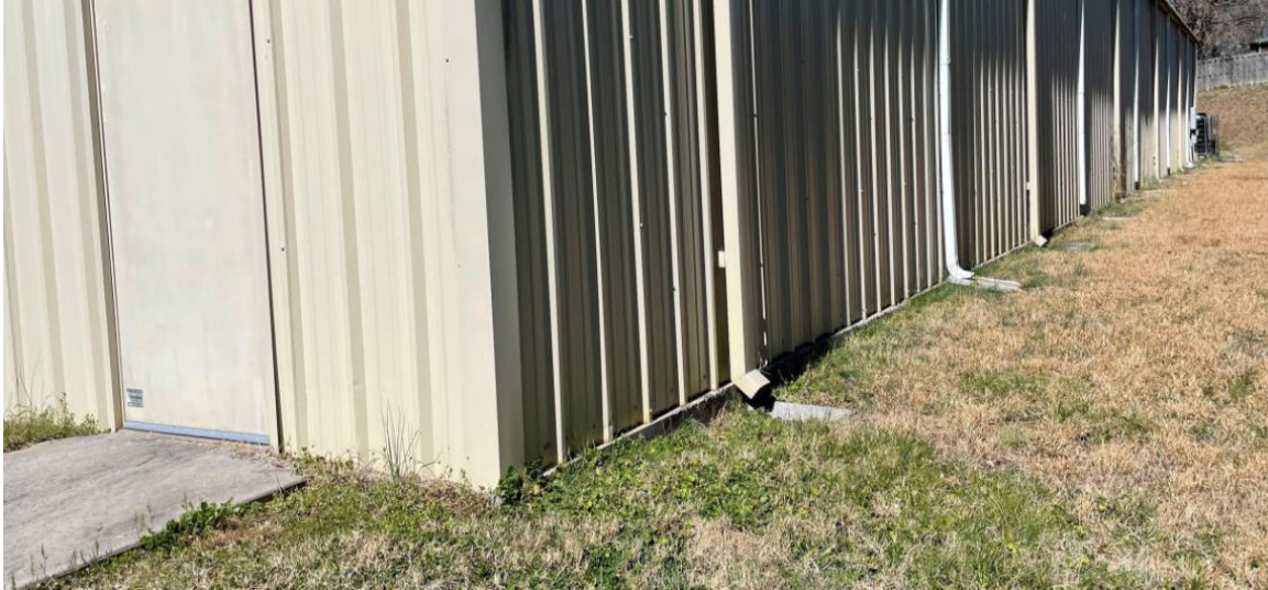
Figure 21 - 2725 Shipetown Rd Dollar General - No 4' planting around 50% of building exterior (there is none on the front or other sides either)
