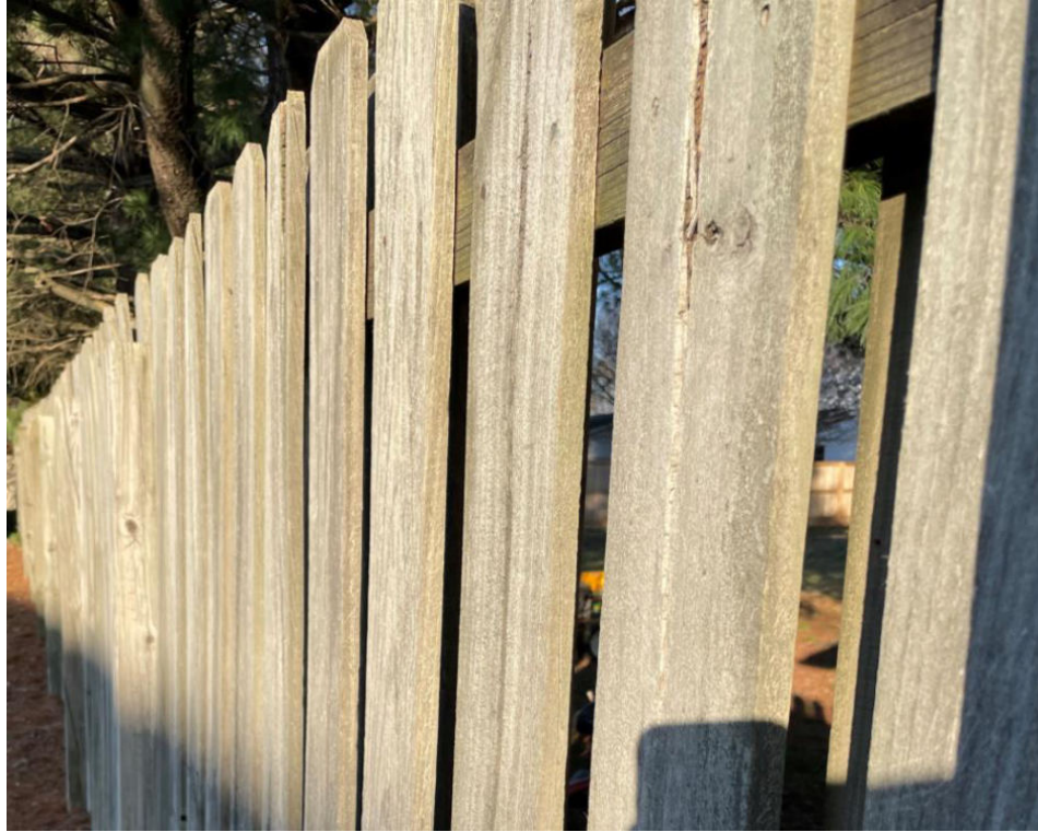
Figure 10 - Privacy Fence between E-Z Stop 1704 W Broadway Ave, Maryville and the adjacent residential lot
