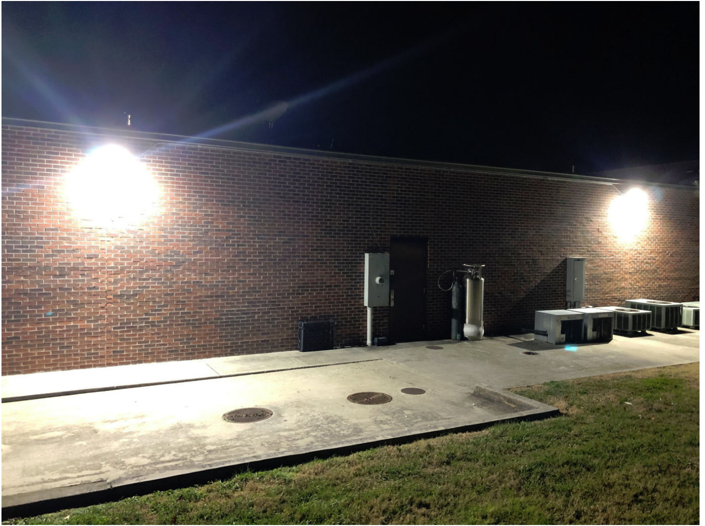
— Wall pack pointed outward, not down - not shielded.jpg
