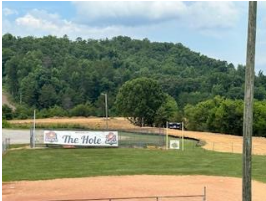
Bower Field has been the site of extensive grading over the past year. (Above, center of image; raw dirt area is new fill)
