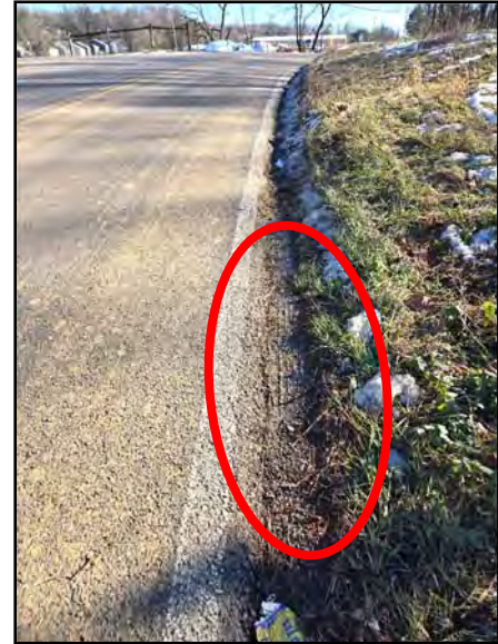
Vehicle Off-Tracking on Amherst Road near Bradley Lake Lane (Looking South)
