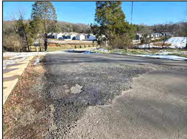
Roughshod Pavement on Bradley Lake Lane near Amherst Road
