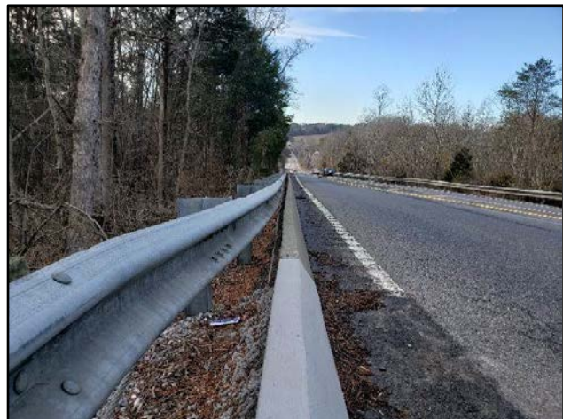
Guardrail and Detached Concrete Curb on South Side of Oak Ridge Highway near Pebblepass Road (Looking West)
