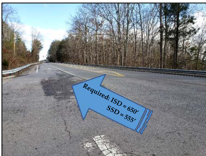
View of Sight Distance on Oak Ridge Highway at Pebblepass Road (Looking East)
