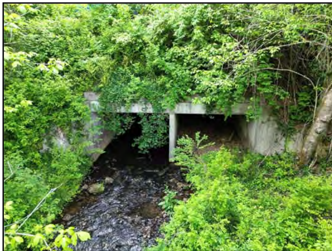
Double-Barrel Concrete Box Culvert over Mill Branch Creek at Proposed Entrance Location
