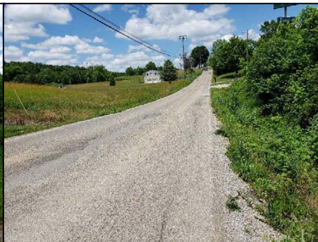
Steep road/shoulder drop-off and deteriorated pavement near 701 Brakebill Road Driveway (Looking North)
