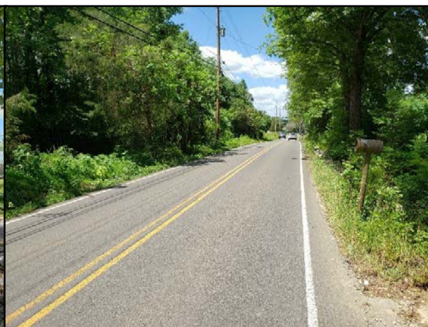
Large trees and utility poles adjacent to the roadway near 508 Brakebill Road with shoulder drop-off into the drainage ditch (Looking North)
