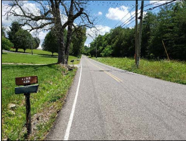
Large trees and utility poles adjacent to the roadway near 428 Brakebill Road with shoulder drop-off into the drainage ditch (Looking South)
