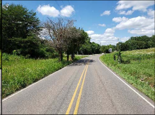
Large trees adjacent to the roadway just south of Kilbridge Drive with shoulder drop-off into the drainage ditch (Looking North)
